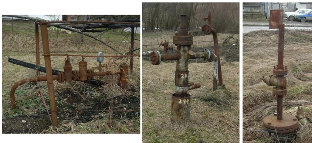
Fig. 3. Modern state of technological oil-extracting equipment of the Skhidnytsya field.
