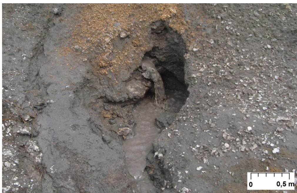
Fig. 1. Brine leakage out of the salt dump No. 1 on the day surface, followed by runoff into the river system and the infiltration into the Quaternary aquifer
